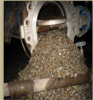
Quagga Mussels on Penstock Belly Drain - Hoover Dam
